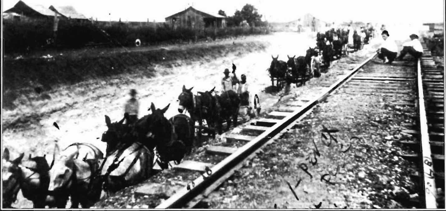
The Bowers Construction Company did the roadbed and tracklaying work on the Bartlett-Florence. Tracks were completed to Jarrell in March 1910. After the B-F was sold to the Bartlett Western, the company finished laying tracks to Florence by the end of 1911.
